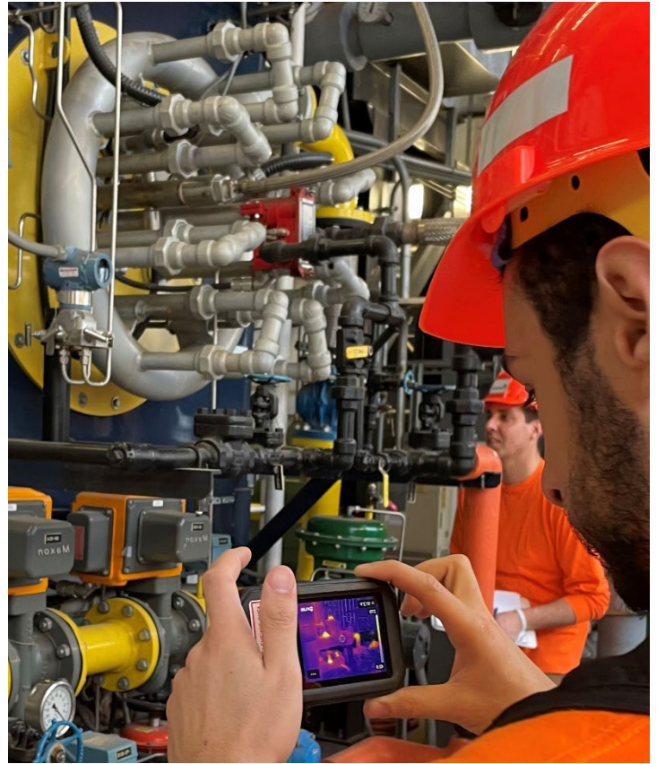
Figure 1: Assessment of Natural Gas Boilers
