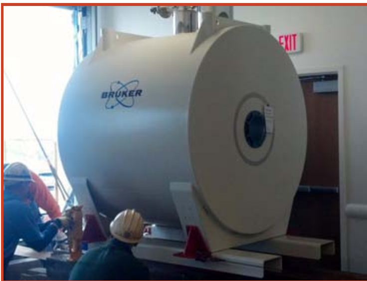
The magnet has just been lifted through a seventh floor door on the east side of the CTRC
