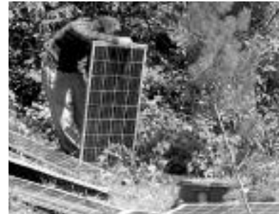
Dave Roberts hooking up solar panels at the Northern Wisconsin field site, Summer 2006. Photo by Mike Loranty.
