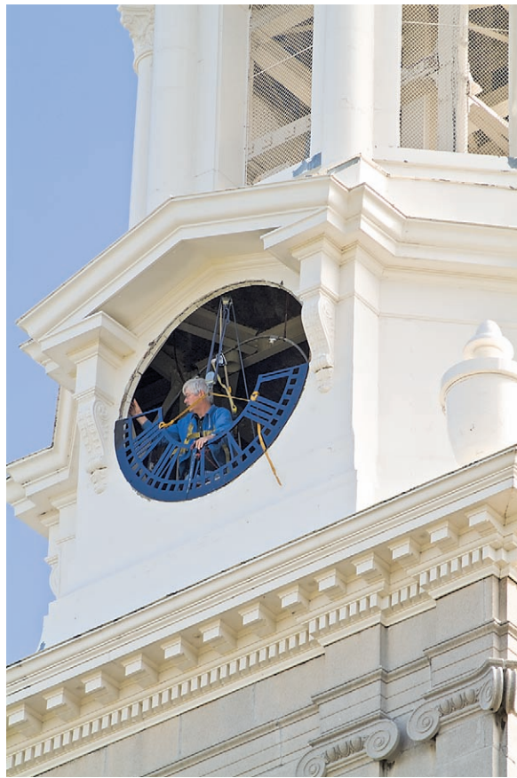
Michael Kuyt of the American Tower Clock Company works on the Hayes Hall clock tower as part of the recent restoration effort.
