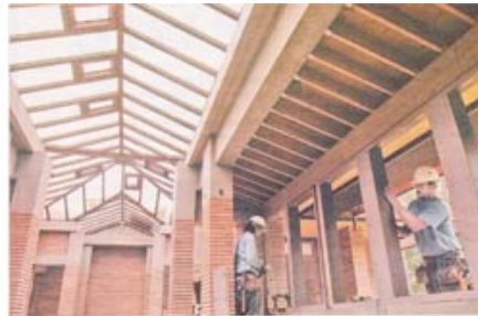
Derek Gee/Buffalo News Workers install the window frames on the east side of the conservatory at the Martin House Complex.
